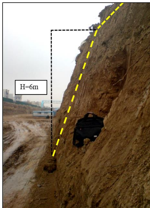
Fig. 8. The stable excavation wall with the approximate depth of 6 m and 80° in zone D 1
